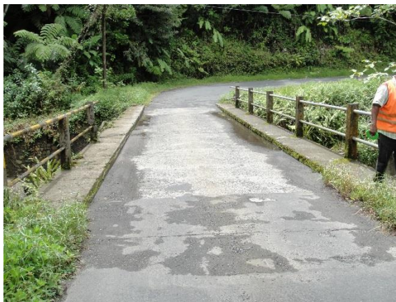
Figure 7 – Missing railings to narrow single lane bridge
