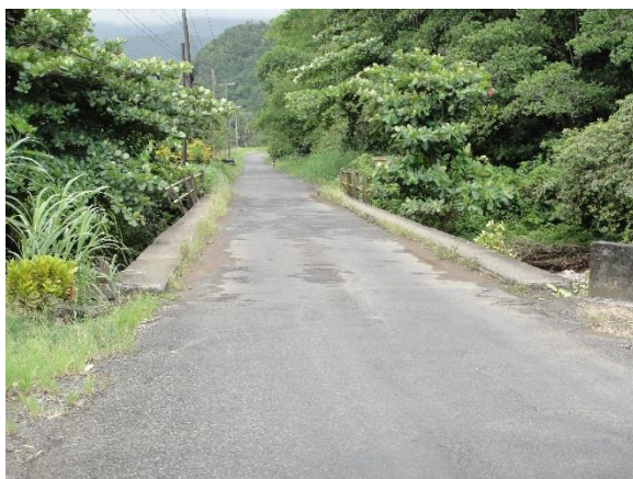
Figure 9 – Damaged safety rails to bridge
