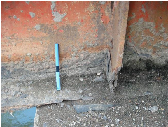
Figure 19 – Corrosion to steel girders of bridge
