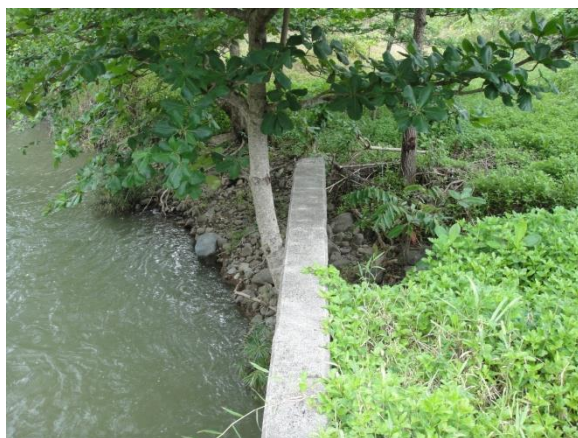
Figure 13 – Both upstream and downstream abutments flanked/scoured
