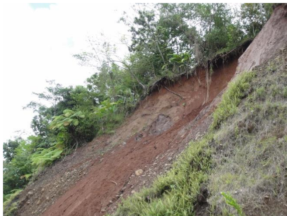
Figure 17 – Unstable slopes at San Sauveur
