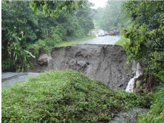
Figure 4 – Resulting gap in road caused by failure of culvert
