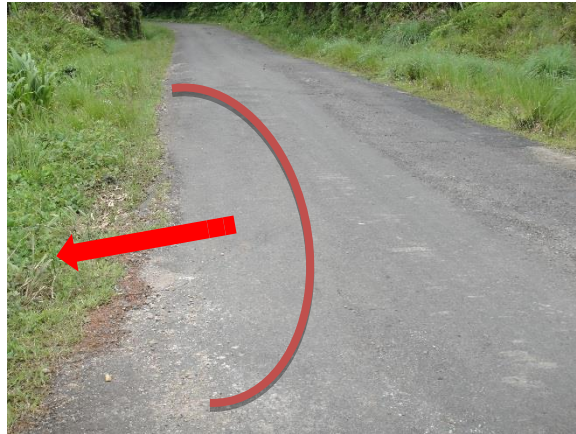
Figure 6 – Subsidence in road showing direction of movement
