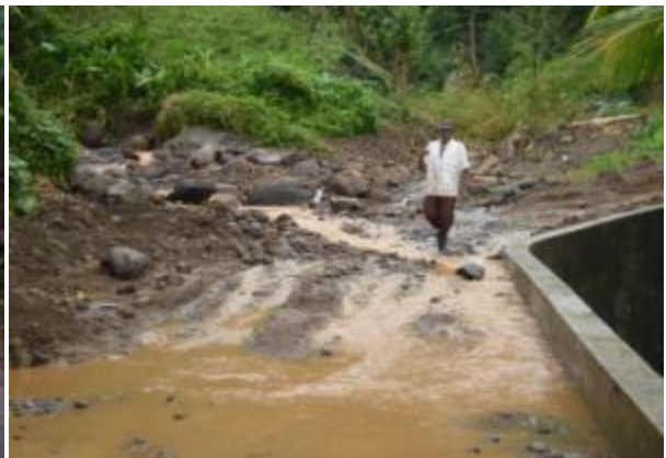
Figure 14: Flooding of culvert structure at Petite Soufriere
