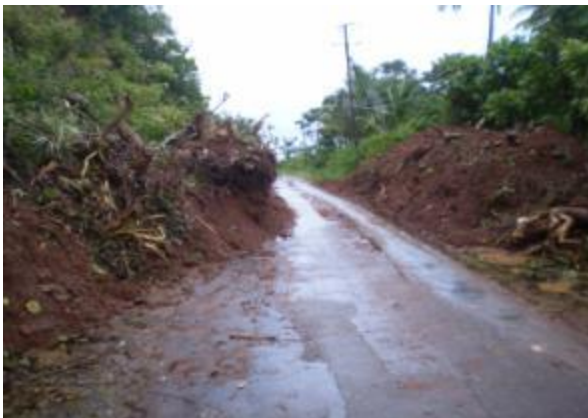
Figure 13: Land Slippage approaching GoodHope Village
