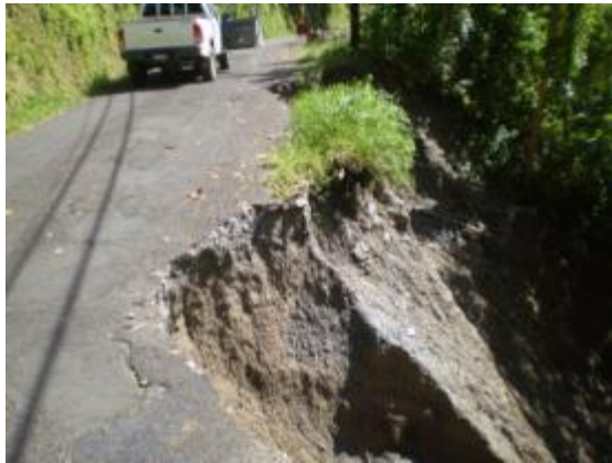
Figure 29: Road edge failure Grand Fond village
