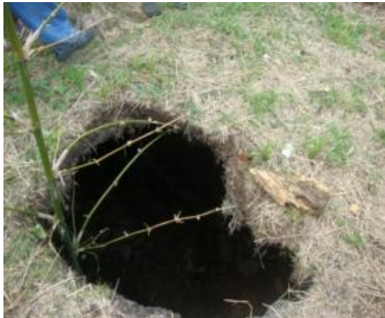
Figure 5: Subsidence above culvert on Fie Road
