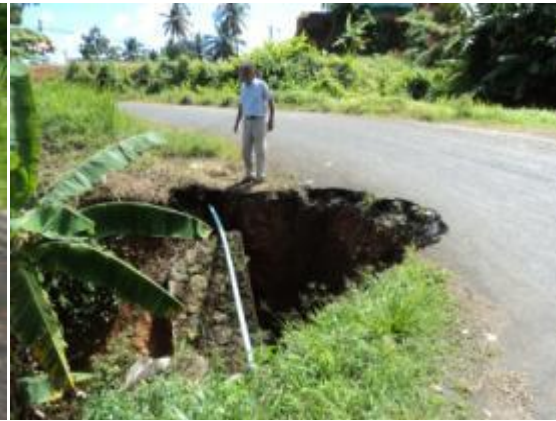
Figure 19: Culvert failure along Carib Territory Road
