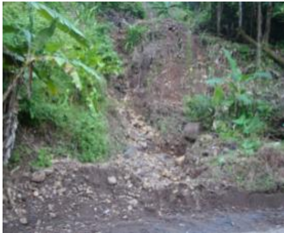
Figure 7: Culvert Blockage and complete cover of inlet on San Sauveur to Petite Soufriere Road
