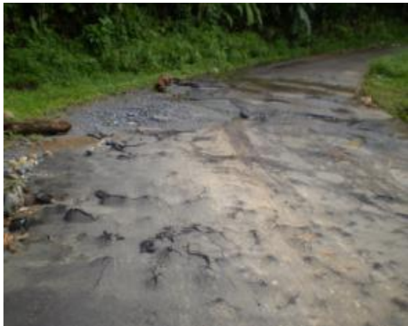
Figure 23: Road Failure at Aux Delices due to flooding.
