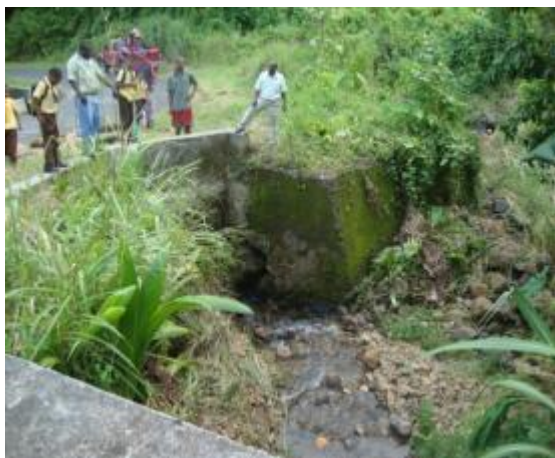
Figure 6: Hole in Culvert Wing Walls on Fie Road
