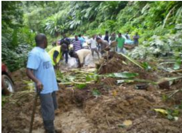
Figure 20: Clearing of mud slide along Bois Diable/Castle Bruce Road
