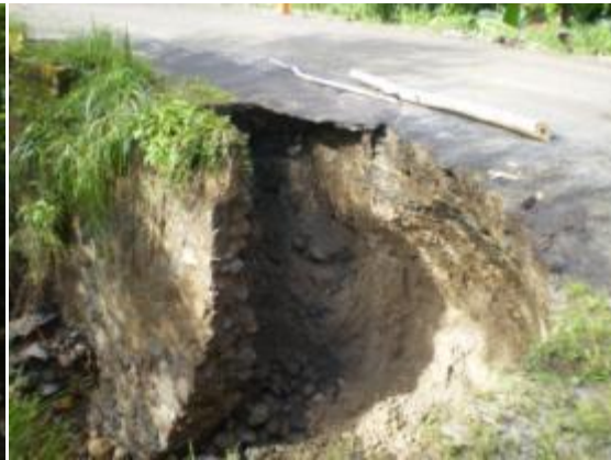
Figure 30: Edge failure Fueyal
