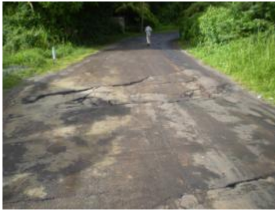
Figure 18: Major road settlement at Mahaut River
