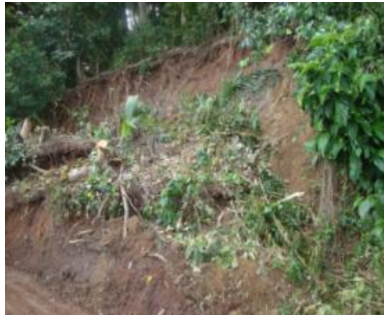
Figure 2: Second Landslide on Jalousie Road
