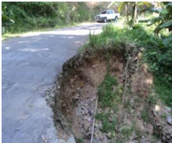
Figure 26: Road edge and Culvert Failure
