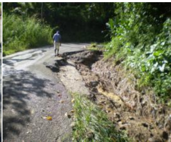
Figure 32: Road edge failure and drainage system
