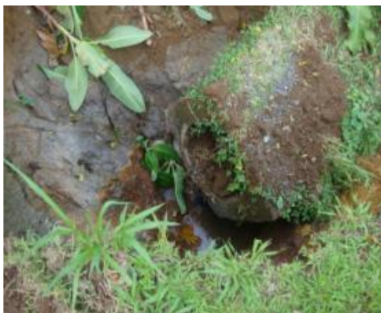
Figure 3: Culvert Failure and Drain Sourcing at Wind Blow Road
