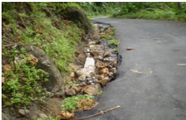
Figure 25: Road edge Failure at Aux Delices
