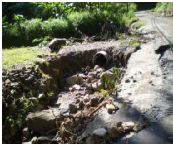
Figure 31: Flooding destroyed road edge and drainage system.
