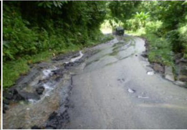
Figure 22: Road /drainage failure at Aux Delices
