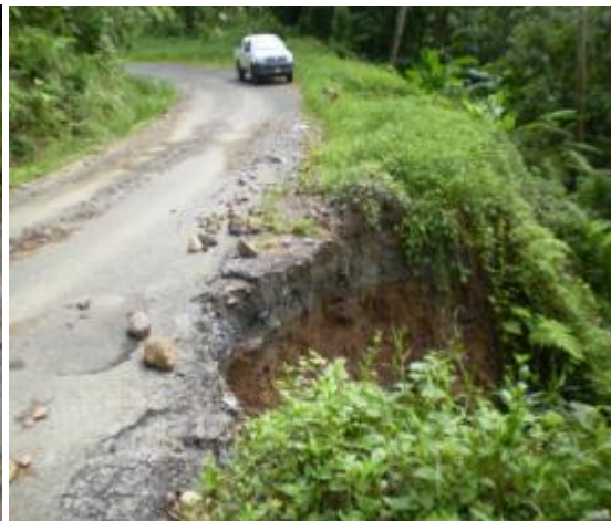
Figure 24: Edge and culvert failure at Aux Delices
