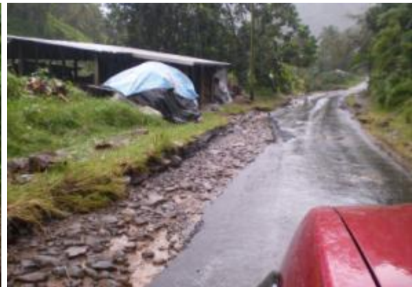
Figure 12: Road edge Failure and Drainage at San Sauveur
