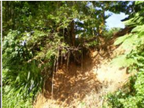
Figure 28: Slope failure at Morne Jaune/Riviere Cyrique
