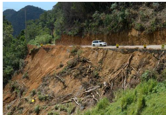
Major landslide on Imperial Highway
